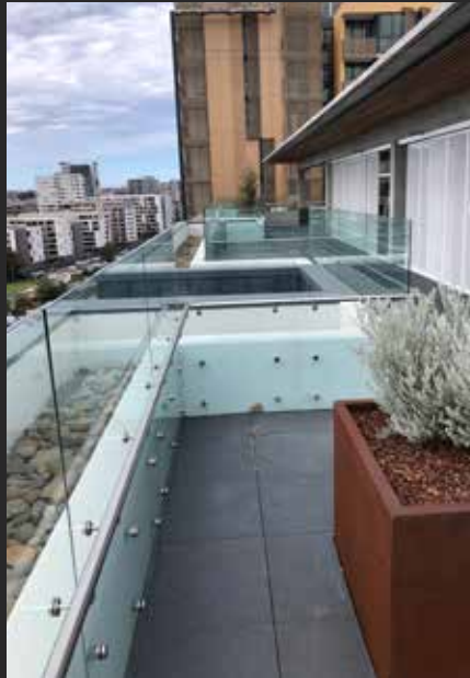
Standoff frameless glass with Stainless Steel Handrail
